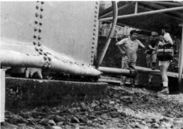
FIGURE 6.13 Circumferential buckling and pipe pullout of the water tank at the Salado pump station.
