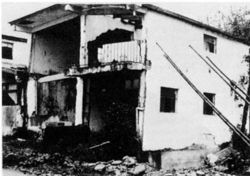
FIGURE 7.2 Damaged concrete-block dwelling in Baeza, Napo Province.
