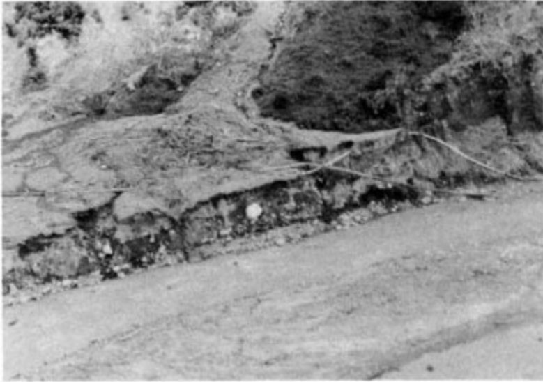
FIGURE 6.8 Trans-Ecuadorian and Poliducto (white) pipelines ruptured by debris flow and deep erosion along the Coca River.
