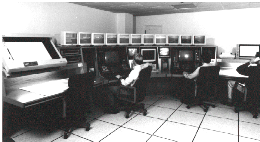
FIGURE 4-2 Control and monitoring station.
