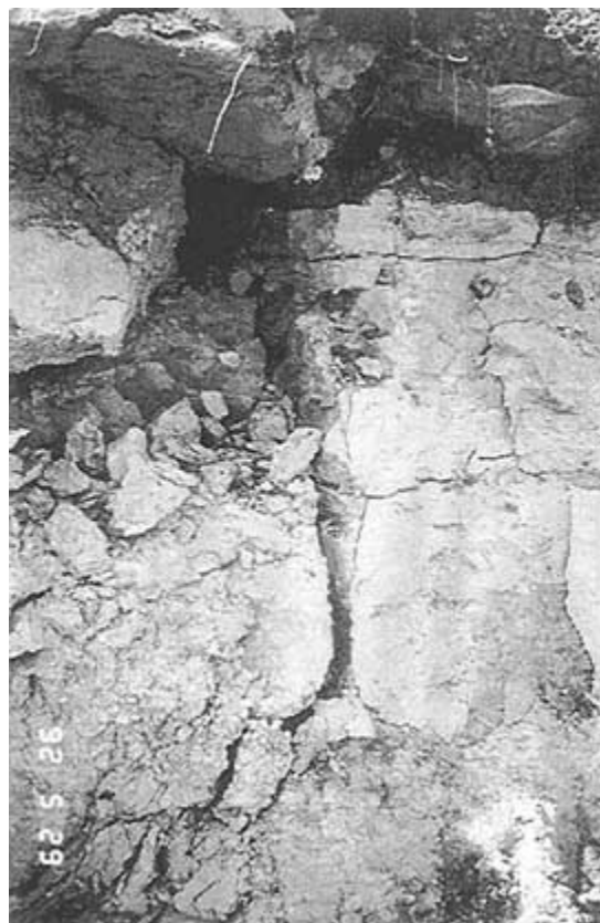
FIGURE 4 Desiccation Crack in Cap Designed as a Resistive Barrier
