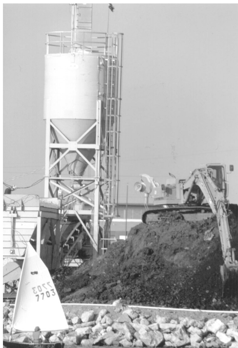
A former fuel storage and handling facility in California was demolished to make way for a marina. As part of the process, 13,000 m 3 of petroleum-contaminated soils were treated in above-ground bioremediation cells. Courtesy of Fluor Daniel GTI.
