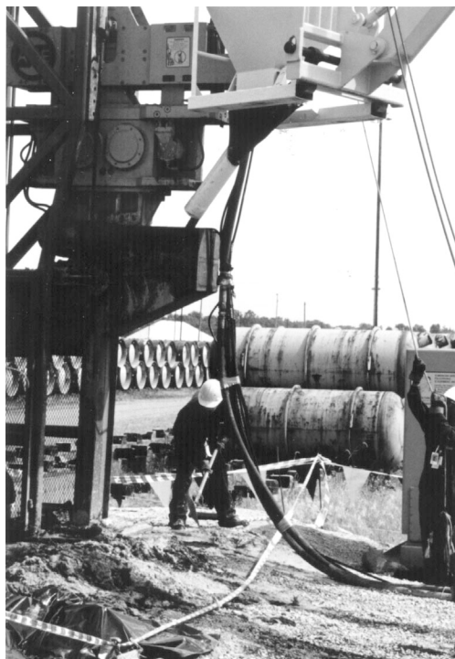
Installing electrodes and treatment zones for a pilot test of electro-osmosis treatment at the Paducah, Kentucky, Department of Energy site. The pilot test was conducted by the Lasagna Consortium™. Courtesy of the Department of Energy.
