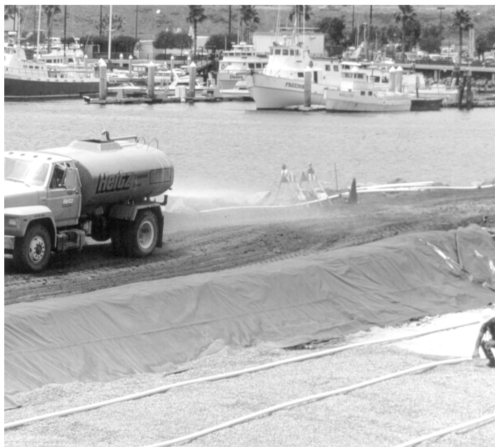
In above-ground bioremediation cells (under construction), oxygen is supplied to soil via a network of embedded piping. Courtesy of Fluor Daniel GTI.
