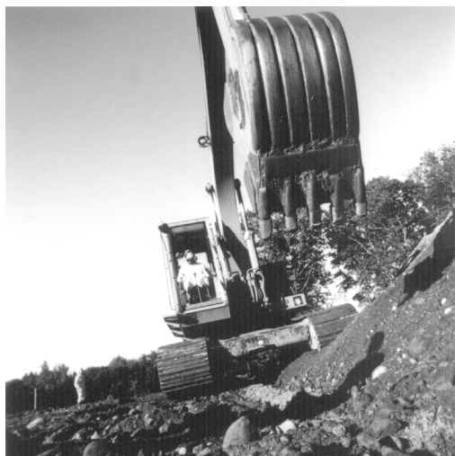
Excavation of soil at a contaminated site. Courtesy of Fluor Daniel GTI.
