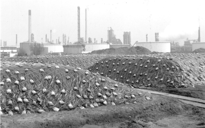
Petroleum-contaminated soils being treated in above-ground bioremediation cells engineered with vapor extraction systems. Courtesy of Fluor Daniel GTI.
