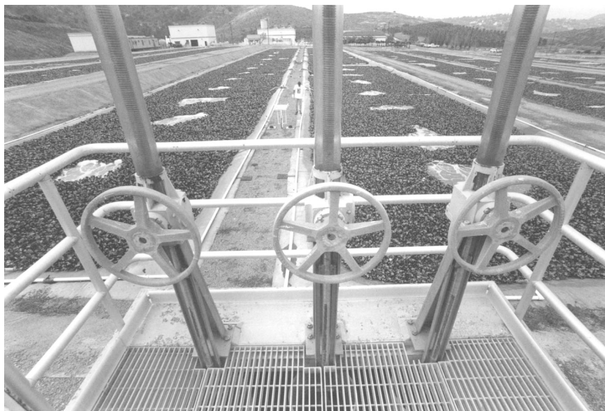
Channels containing water hyacinths, used to provide secondary treatment at San Diego's Aqua II pilot facility. Photo by Joe Klein.
