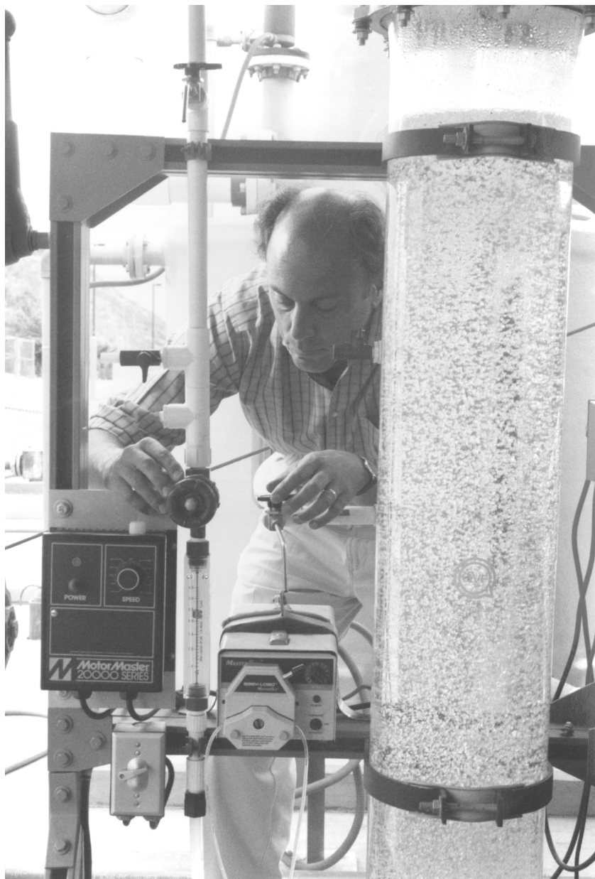
Checking the ozone disinfection unit at San Diego's Aqua III water reclamation facility. Photo by Joe Klein.
