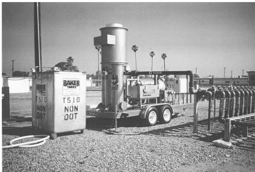
This Soil Vapor Extraction Treatment System is being used for removing petroleum vapors from the underlying vadose zone above the ground water aquifer. Courtesy of the U.S. Navy.
