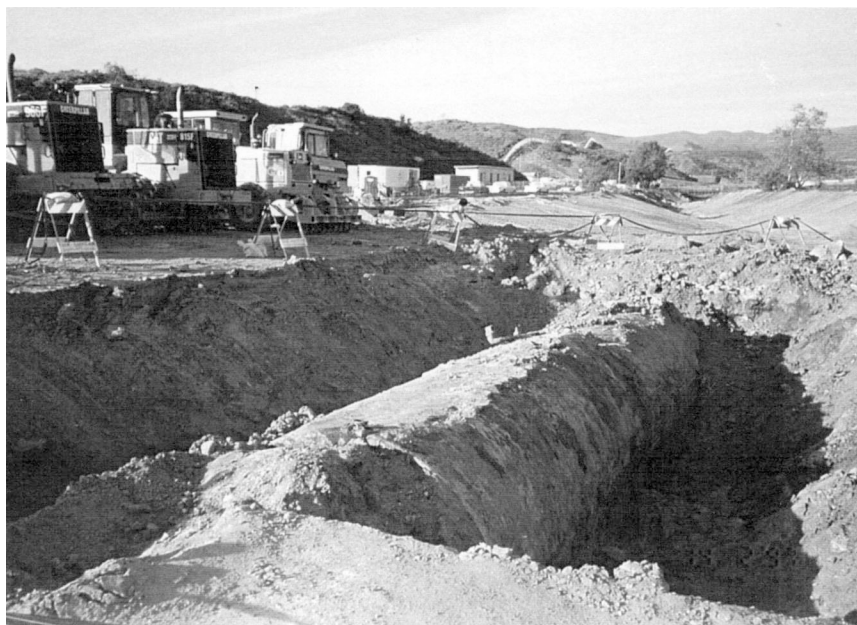
The excavation of two inactive underground storage tanks is one of thousands taking place at Navy facilities across the country. Courtesy of the U.S. Navy.
