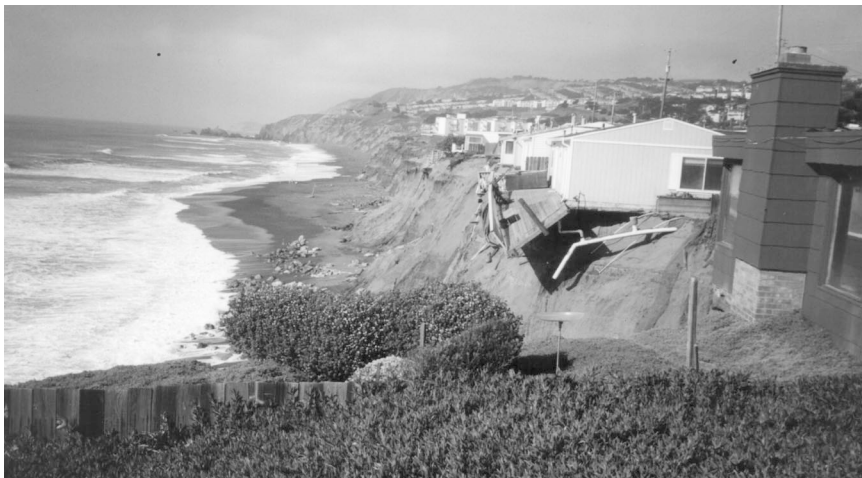
Bluffs cut away by damage from El Niño storms in Santa Cruz, California, March 1998. Courtesy of Monty Hampton, U.S. Geological Survey, Menlo Park, California.
