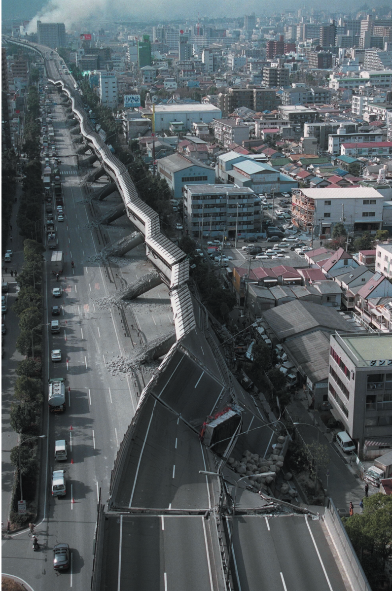
FIGURE 1.1 Scene of destruction in Kobe, Japan, from the 1995 Hyogo-ken Nanbu earthquake (magnitude 6.9), showing a collapsed section of the Hanshin Expressway. This event killed at least 5500 people, injured more than 26,000, and was responsible for approximately $200 billion in direct economic losses. SOURCE: Pan-Asia Newspaper Alliance.
