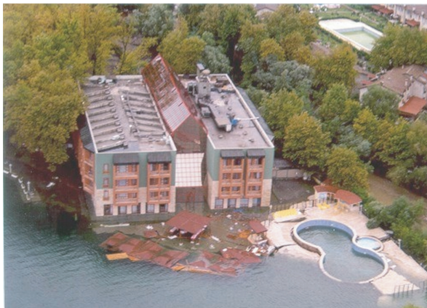
FIGURE 3.5 Many apartment buildings on the fringe of the river delta at Golcuk, Turkey, slid into the sea during the Izmit earthquake of August 17, 1999. Land-use planning that accounts for the instability of young deltaic sediments could substantially reduce loss of life and property in future earthquakes. SOURCE: A. Barka, Istanbul Technical University.
