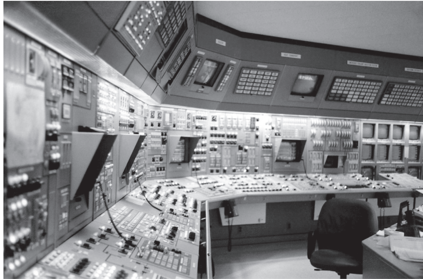
FIGURE 1 A typical control room for a nuclear power plant. Source: Photo courtesy of C.M. Burns.
