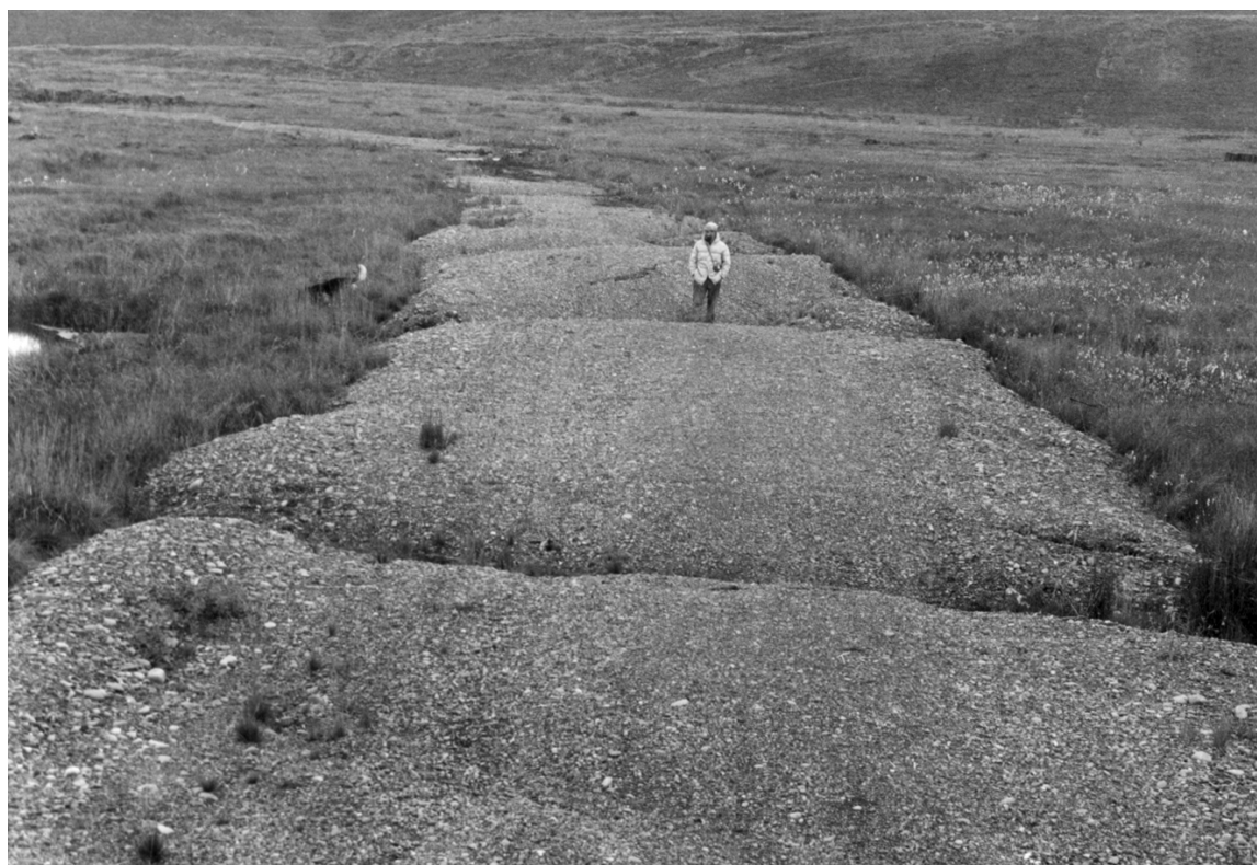
FIGURE 6-4 Roadway destroyed by thawing ice edges near Umiat. Gravel fill was not thick enough to replace insulating effect of the organic mat, which it destroyed. Photograph by Gordon Greene. SOURCE: Lachenbruch 1966.
