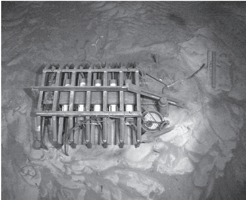
FIGURE 2-2 Seafloor junction box at HUGO, atop Loihi Volcano off Hawaii, after five years on the ocean floor. The partially buried package, recovered in October of 2002, is still in excellent condition. Use of titanium and plastics has virtually eliminated corrosion problems. Figure courtesy of Fred Duennebier, University of Hawaii.
