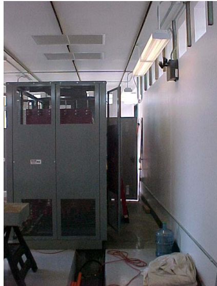
FIGURE 10 TriMet Interstate MAX LRT Expo Substation, 2003.
