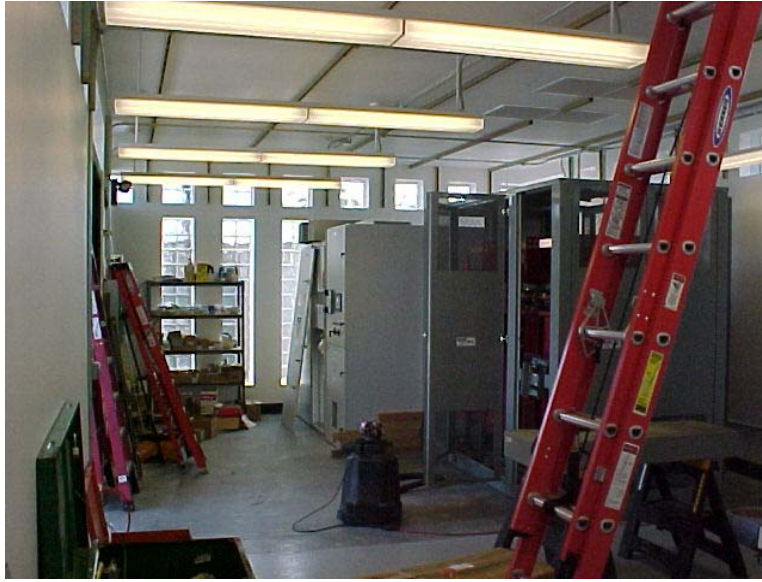
FIGURE 9 TriMet Interstate MAX LRT Expo Substation, 2003.
