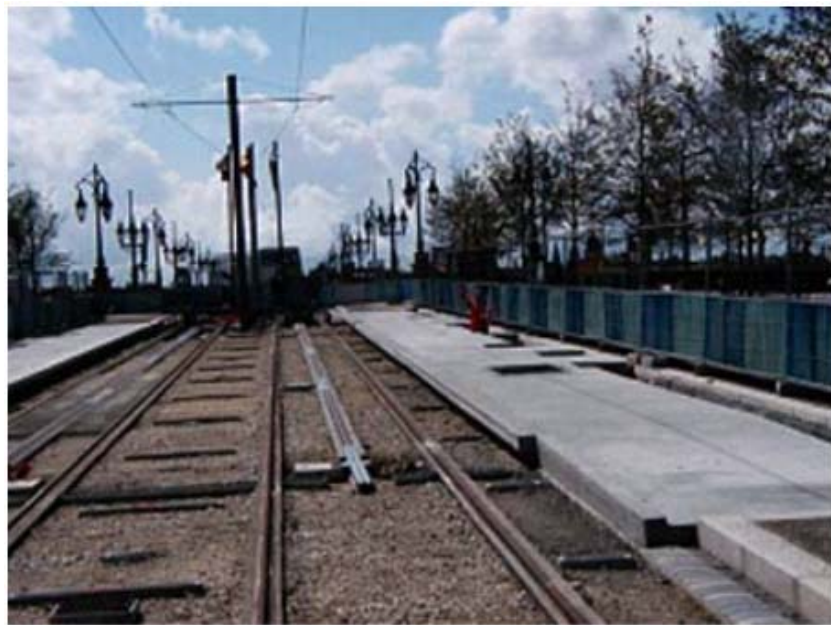
FIGURE 6 Station transition point.
