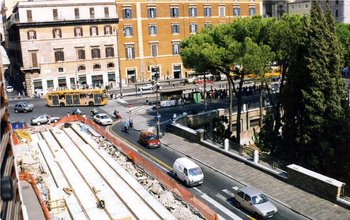
FIGURE 11 Side and central precast concrete slabs have been laid and joined to the precast concrete platform in Piazza di Torre Argentina.
