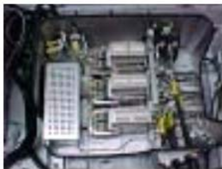
FIGURE 18 Power control box.
