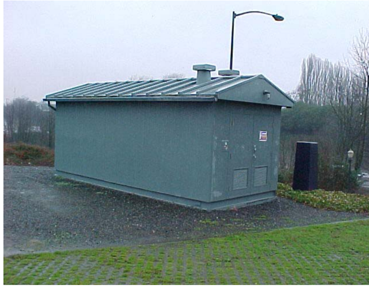
FIGURE 1 TriMet Banfield LRT Project Lloyd Center Substation, 1986.
