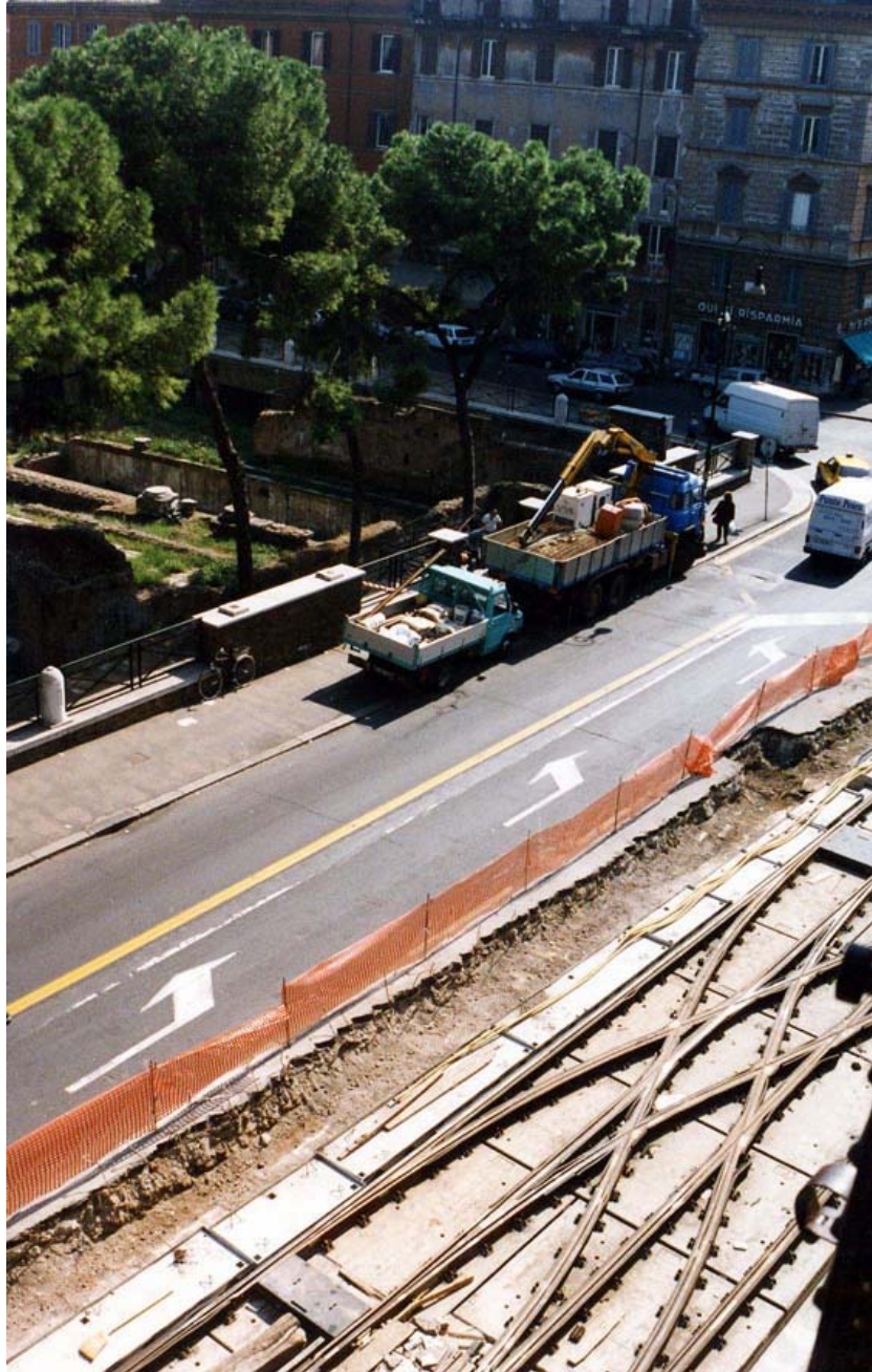
FIGURE 10 Piazza di Torre Argentina: tracks have been laid upon the precast concrete platform near Roman monuments dating back to the 3rd century B.C.
