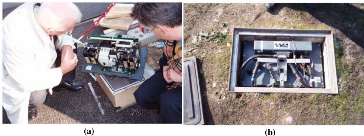
FIGURE 13 (a) Interior of power rail control unit; and (b) Installed power rail control unit.
