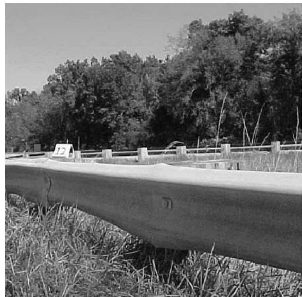
Figure 7. An example of minor guardrail damage.
