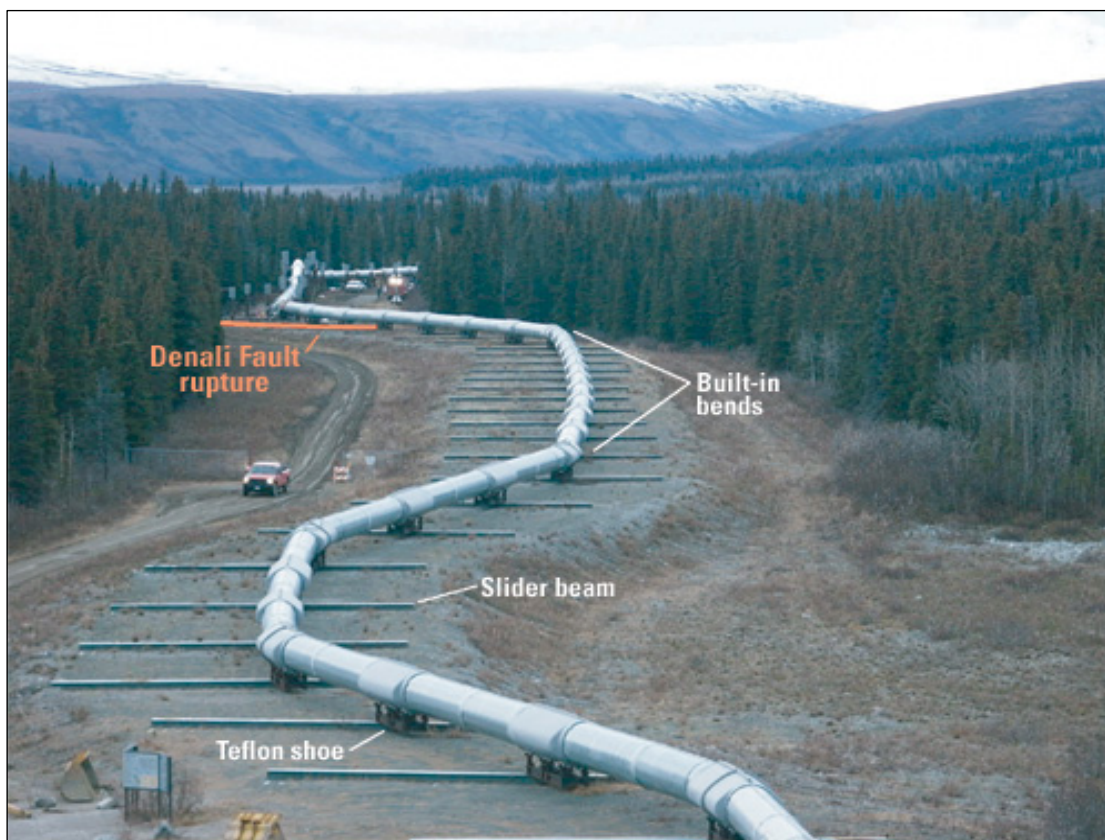
FIGURE 1. The Trans-Alaska Oil Pipeline, built in the 1970's, crosses the Denali Fault in Alaska. During the 2002 Denali Fault quake, magnitude 7.9, the ground was offset beneath the pipeline, and violent shaking damaged a few of the pipeline's supports near the fault, but the pipeline did not break. (Source: Kathy Olsen, OSTP).
