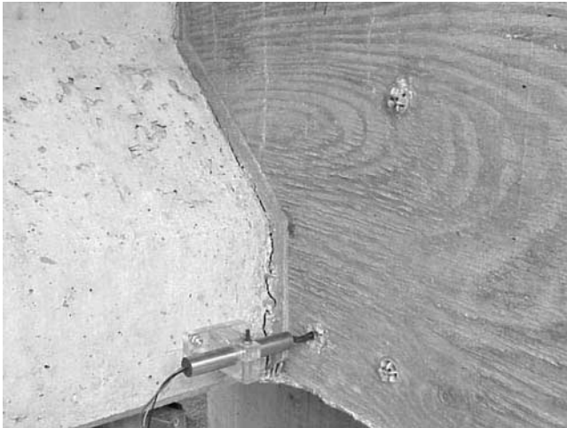
Figure 56. Crack at bottom of girder after post-tensioning and shimming.
