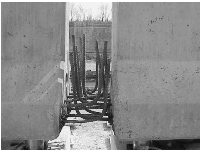
Figure 30. Misaligned bars due to field bending.
