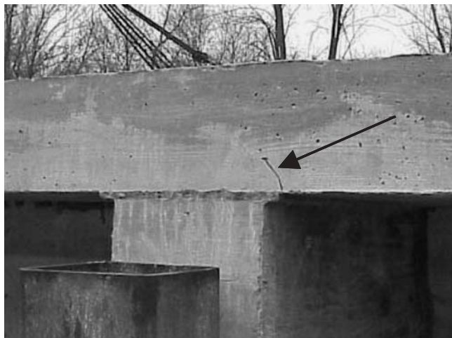
Figure 58. Slab cracking in full-size Specimen 2.
