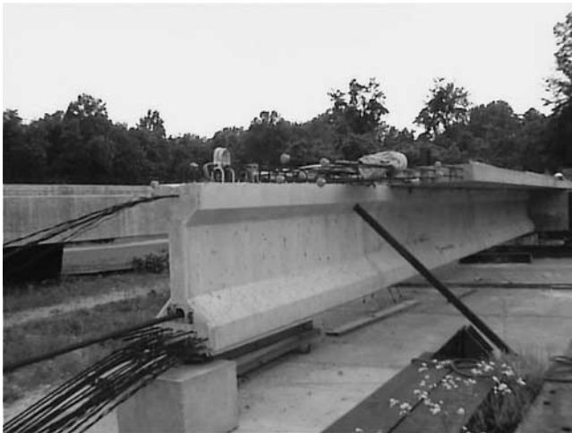
Figure B-13. End of Specimen 1 showing extended bar, extended strand, and post-tensioning bar.
