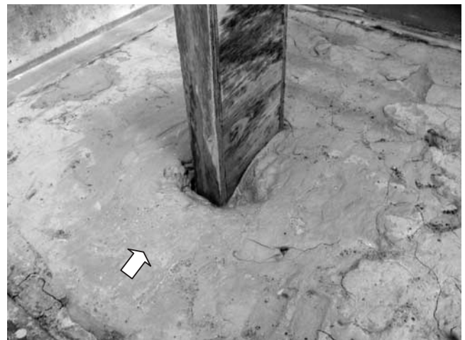
Figure A12 Scour Hole in Test Sh-3.
