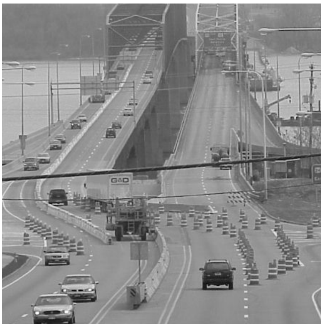
FIGURE 50 West entrance of the McClugage Bridge construction zone reversible segment, Peoria, Ill. ( Source : "Fact Sheet 5—Innovation During Bridge Rehabilitation Improves Mobility" 2003).
