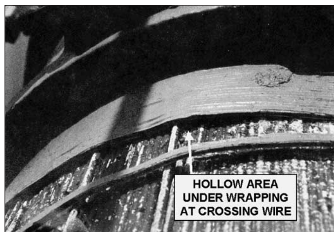
Figure 2.3.1.2.2-4. Hollow area indicating crossing wires.
