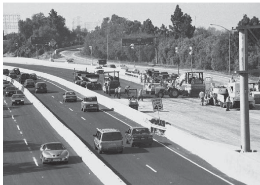
Nine-inch overlay of polymer-based asphalt laid on I-710 was specifically designed both to carry the projected traffic loads and to last 30 to 40 years with minimal maintenance.
