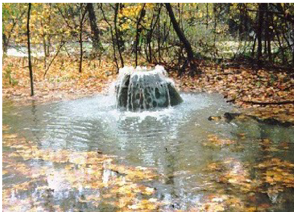
FIGURE 4-6 Sanitary sewer overflow from an elevated manhole in the Pittsburgh region. SOURCE: Photograph courtesy of 3RWW.
