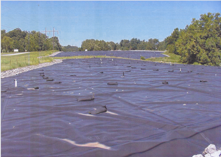
FIGURE 4.1 Trench caps made of high-density polyethylene (HDPE) are expected to last at least one hundred years. There are no field data to confirm this expectation, rather experience has shown punctures, tears, and deformations. Photo courtesy of Oak Ridge Operations Office.
