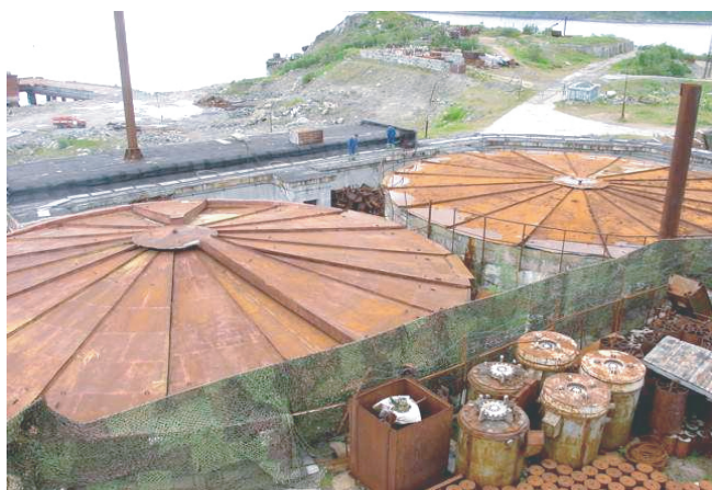
FIGURE 15 View of the rooftops of Buildings 2A and 2B of the spent nuclear fuel dry storage facility at the Andreeva Bay base.
