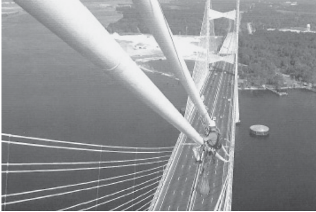
FIGURE 56 Rolling device for inspection of the stay cables on the Dame Point Bridge (“B&N Creates Custom Device . . .” 2005).
