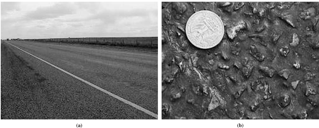
FIGURE 60 (a and b) Results of excess binder—Bleeding in wheel paths.
