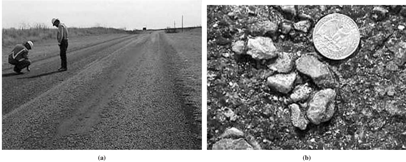
FIGURE 61 (a and b) Results of aggregate loss—Raveling.
