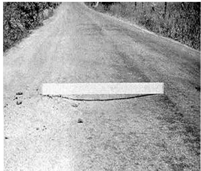
FIGURE 63 Rutting ( Asphalt Surface Treatments—Construction Techniques 1988).
