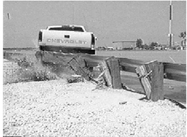
Figure 11. Guardrail damage in TTI Test 404201-1.
