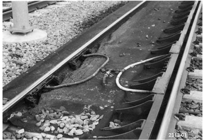
Figure 13. Location receiving both gage face and restraining rail lubrication.
