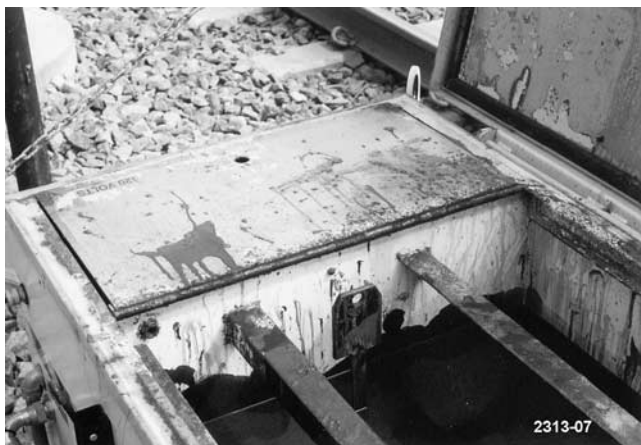
Figure 18. Corrosion of tank components caused by friction control material carrier.
