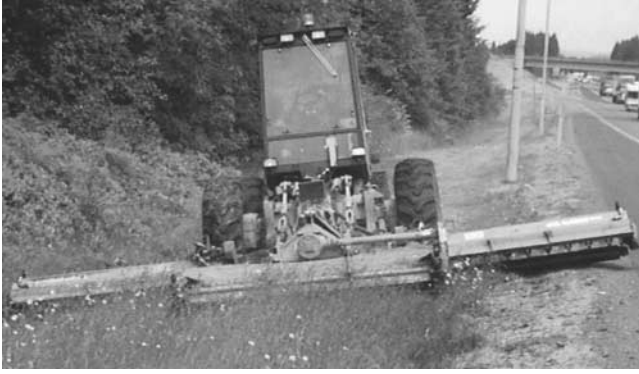
FIGURE 12 Well-planned roadsides, at time of construction or reconstruction, can accommodate integrated vegetation management practices (courtesy: Washington State DOT).
