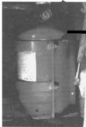
Extinguishing Agent Tank (Dry Chemical)
