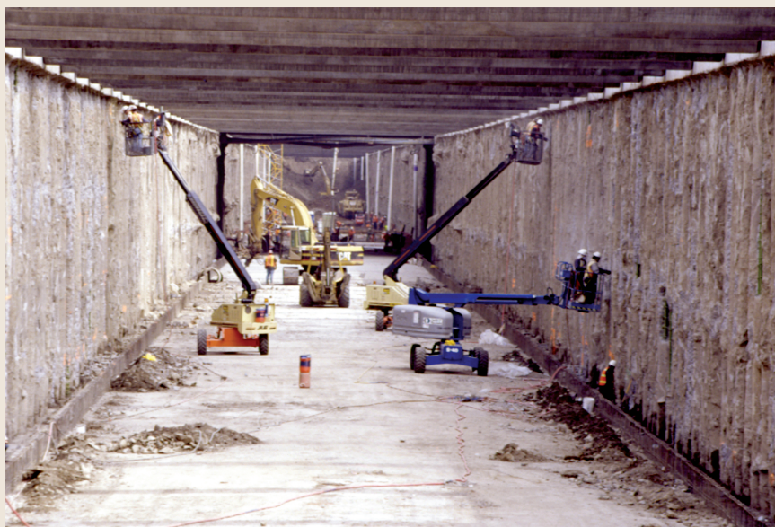
FIGURE: Mid-corridor track construction (image courtesy of the Alameda Corridor Transportation Authority).
