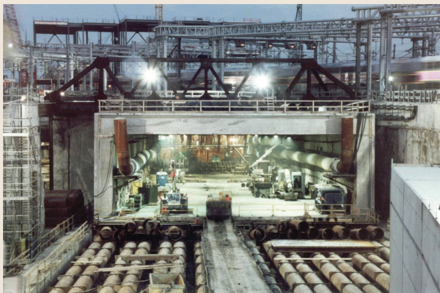
FIGURE: A view of the rear end of the tunnel box being jacked into place for the eastbound lanes of I-90 below the railroad tracks in Boston. A train is visible, passing over top of the tunnel. This jacked tunnel box was 36 feet high, 79 feet wide, and 379 feet long, and weighed approximately 32,000 tons. Used with the permission of the Massachusetts Turnpike Authority.
