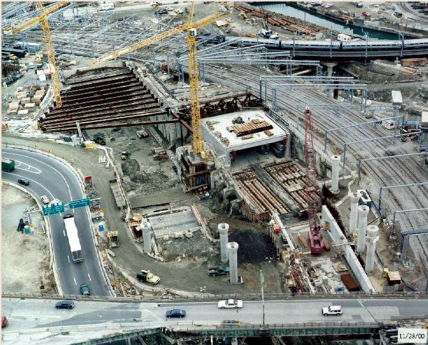
FIGURE: An aerial shot of the worksite in Boston where the tunnel jacking was done, showing the two large pits from which the I-90 westbound tunnel box (left side, with a series of steel struts across the top of the pit to brace it) and the I-90 eastbound tunnel box (pit to right) were jacked. At the time this photo was taken, the westbound tunnel box had been completely jacked into place, while the eastbound tunnel box jacking operation was still in progress. Used with the permission of the Massachusetts Turnpike Authority.
