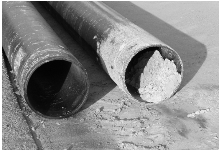
Backfill sand contaminating a new pipe at a water main construction site. Photo courtesy of Bureau of Laboratory Service, Philadelphia Water Department.
