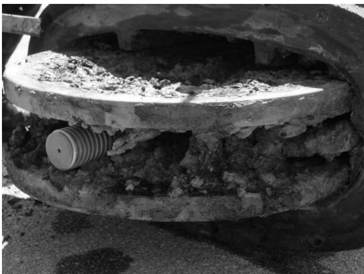
Valves should be inspected and operated on a regular basis to prevent rust and encrustation from interfering with their performance. Photo courtesy of Bureau of Laboratory Services, Philadelphia Water Department.
