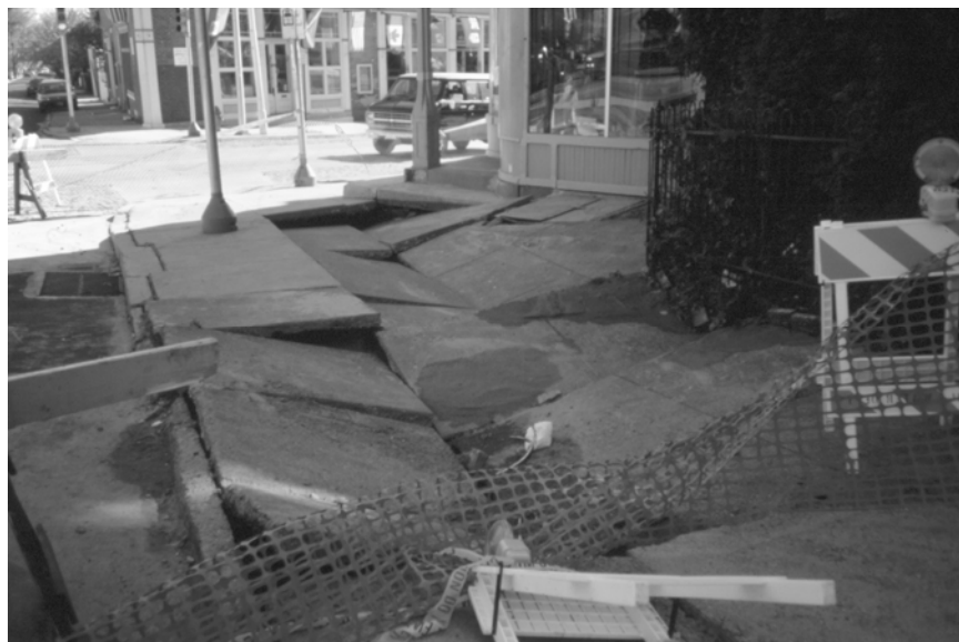
The after effects of a water main break that occurred beneath the side walk of an urban street. Photo courtesy of Bureau of Laboratory Services, Philadelphia Water Department.
