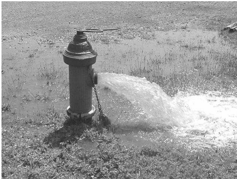
Hydrant flushing. Photo courtesy of Bureau of Laboratory Services, Philadelphia Water Department.
