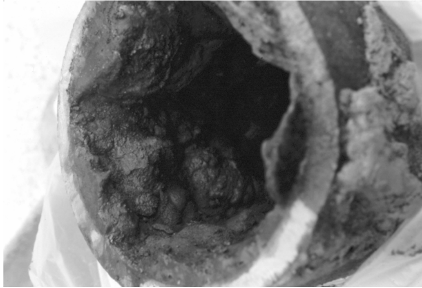
The effects of internal corrosion, shown as a build up of tuberculation, on an unlined cast iron water main. Photo courtesy of Bureau of Laboratory Services, Philadelphia Water Department.
