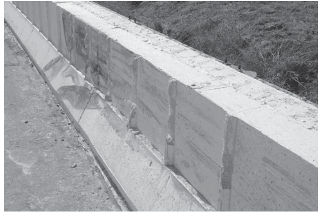
Figure 68. Barrier damage for Crash Test 1.
