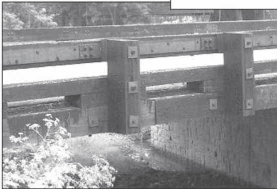
The trim hardware on this concrete bridge deck adds the convincing detail for this deception.
