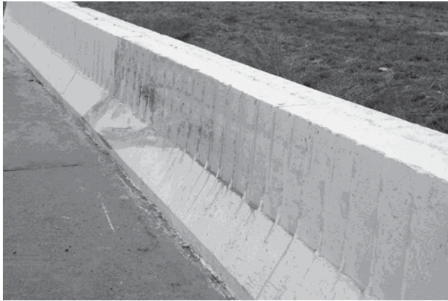
Figure 70. Barrier damage for Crash Test 2.
