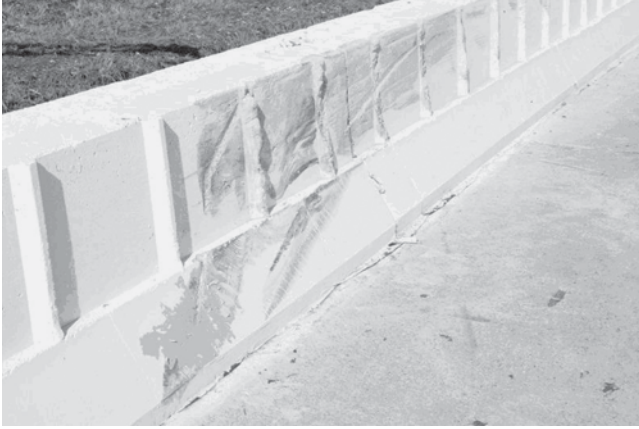
Figure 72. Barrier damage for Crash Test 3.
