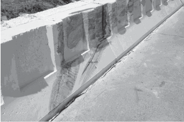
Figure 81. Barrier damage for Crash Test 7.
