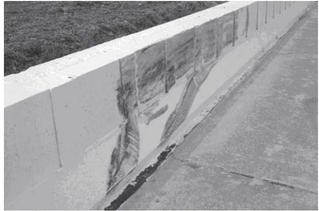
Figure 76. Barrier damage for Crash Test 5.
