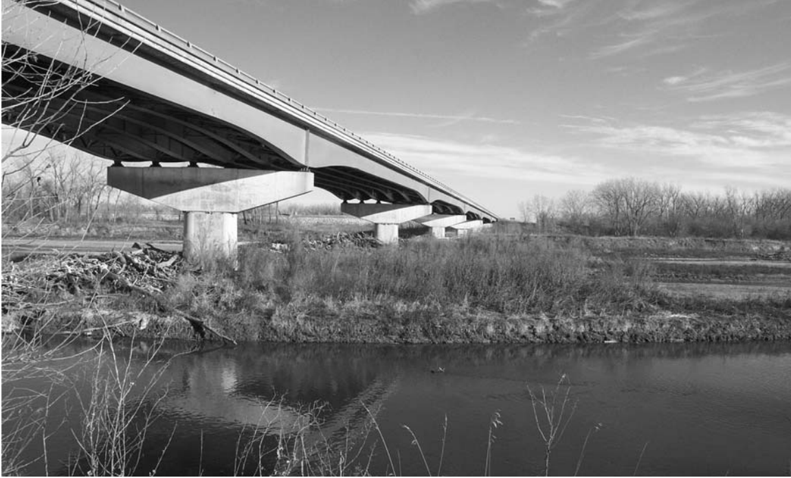
FIGURE D6 K-18 bridge site located on the Kansas River between Manhattan and Junction City.
