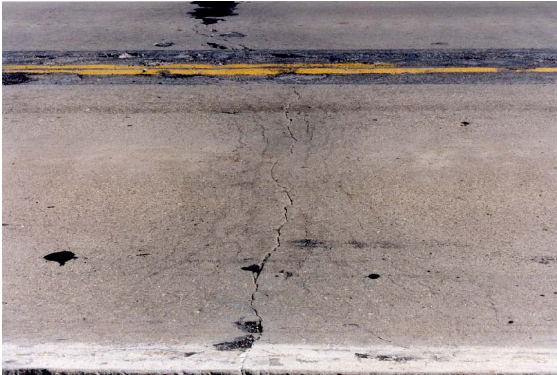
FIGURE 2 D cracking distress at transverse crack.
