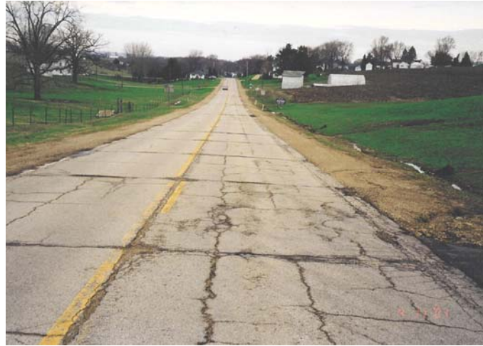
FIGURE 3 Reflection cracking in HMA overlay over PCC pavement. (Photo courtesy of Antigo Construction.)
