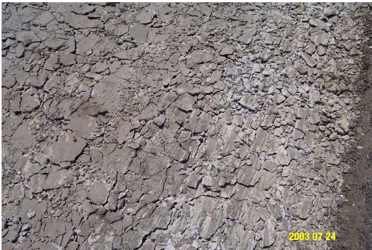
FIGURE 5 Note the “flaky” rubblized PCC surface.
