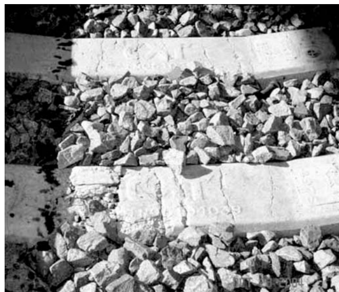
Figure 2 Cracked concrete ties at the abutment of a freight railroad ballast deck bridge caused by impact loads.
