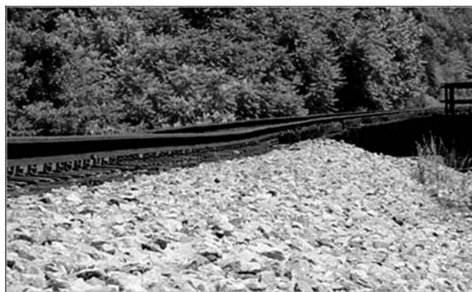
Figure 1 Typical differential settlement of a freight railroad ballasted track bridge approach.
