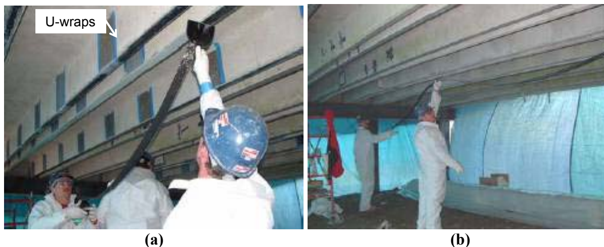
FIGURE 13 Externally bonded FRP: (a) sheets and (b) strips for flexural strengthening of prestressed concrete girders
