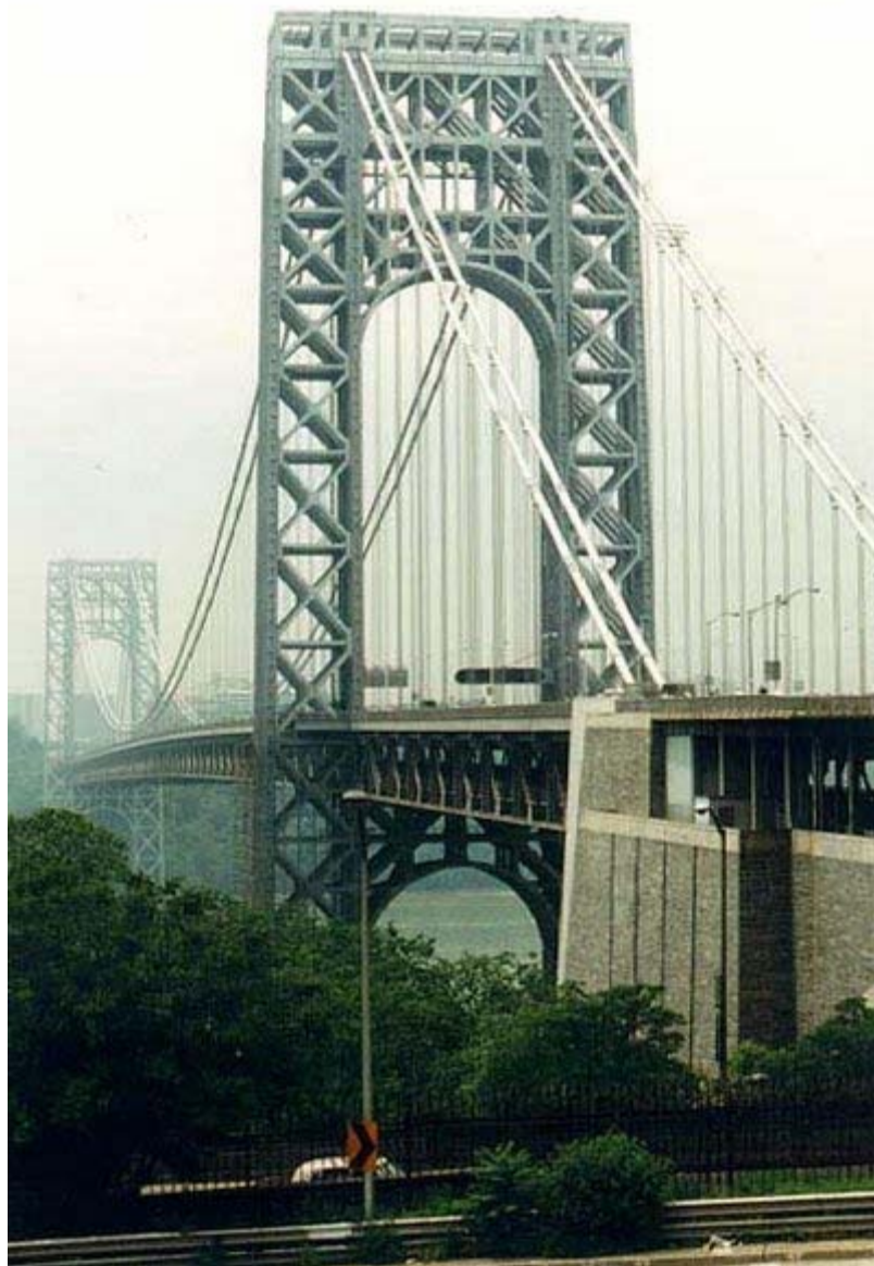
FIGURE 3 The George Washington Bridge, crossing the Hudson River in New York, opened to traffic in 1931. The lower level opened in 1962. In 1981, the bridge was designated a National Historic Civil Engineering Landmark by the ASCE.
