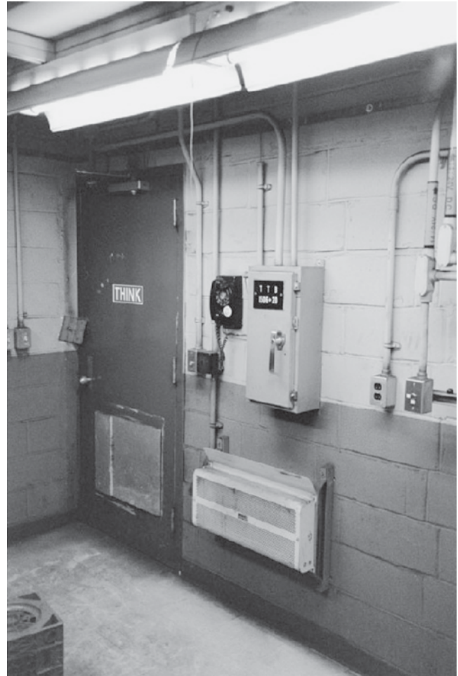
Figure 9 View of interior of relay room for receiver station and data transmission line.
