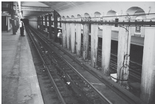
Figure 3 View looking northward of transmitter location midway along 190th Street station. Cables can be seen between the case and rail. The transmitter case is located between pillars, center between tracks.
