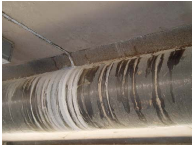
Figure 5.2.1.1-5 Leakage through deck-to-deck joint.
