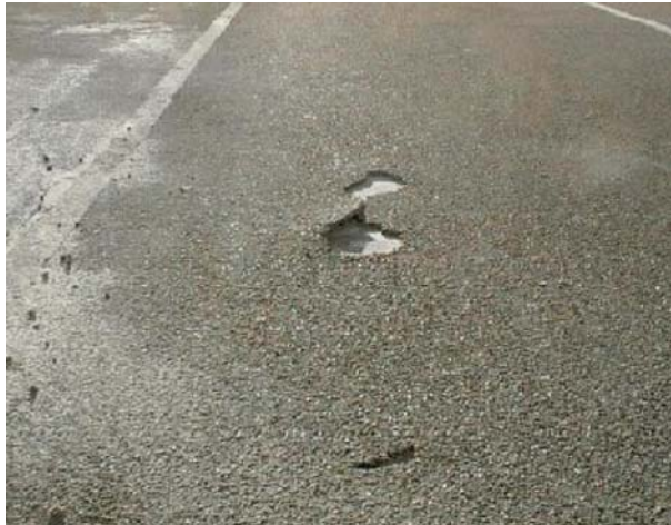
5.2.1.4-2 Wear surface debonding.
