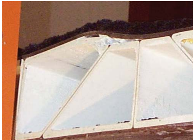
Figure 5.2.2.1-7 Tearing of core leading to facesheet buckling.
