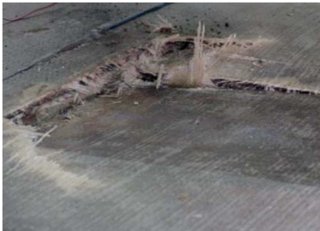
Figure 5.2.2.1-3 Punch-through of the deck from impact (Schuyler Heim Bridge).
