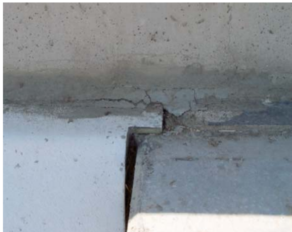
Figure 5.2.1.5-4 Concrete cracking at the parapet-to-FRP-deck interface.
