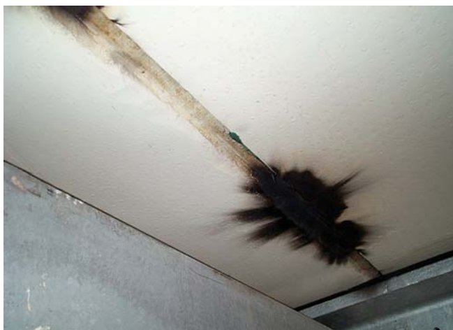
Figure 5.2.2.1-4 Attempted ignition of deck material by vandals.
