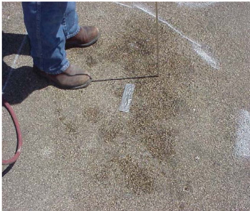
Figure 8-4 Water spouting out of drill holes on deck.
