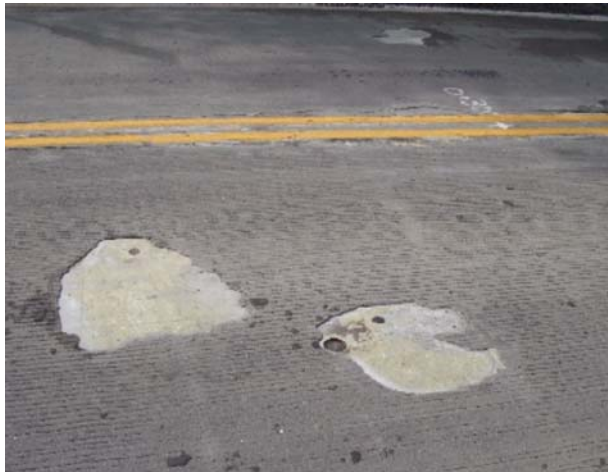
Figure 5.2.1.4-1 Delamination/failure of wear surface on an FRP deck.
