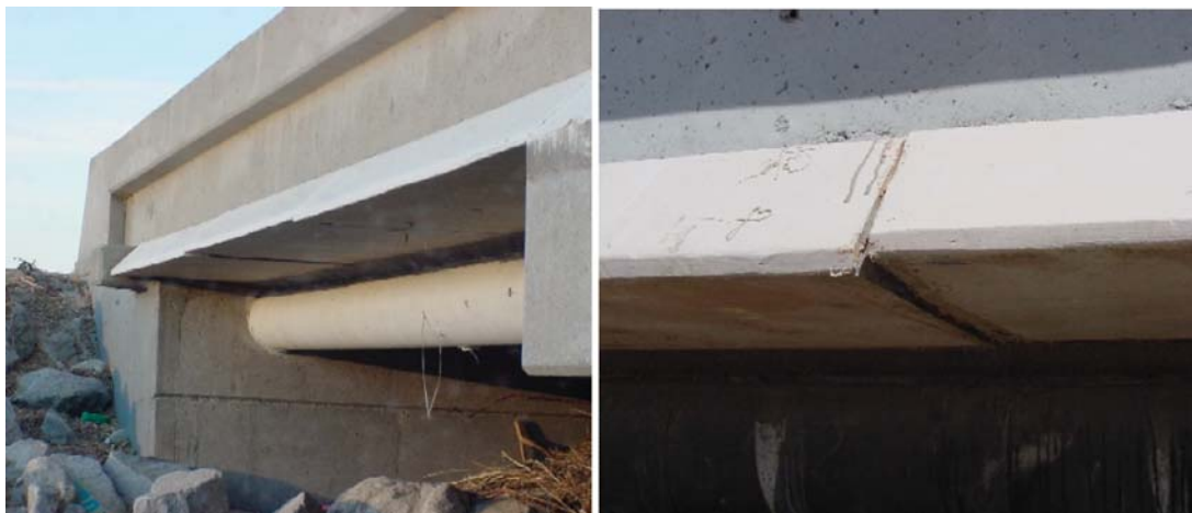
Figure 5.2.1.1-3 Misalignment of deck-to-deck joint.
