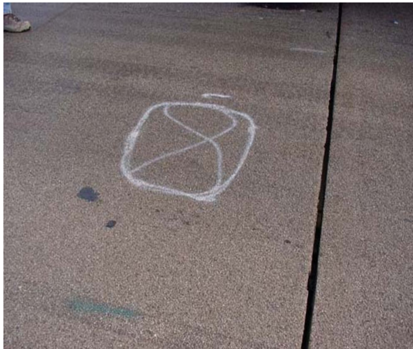
Figure 8-6 Tap tests indicate debonding of facesheet.
