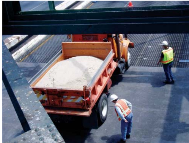
Figure 5.1.1-1 Dump truck placed on deck to reveal any cracks in FRP deck.
