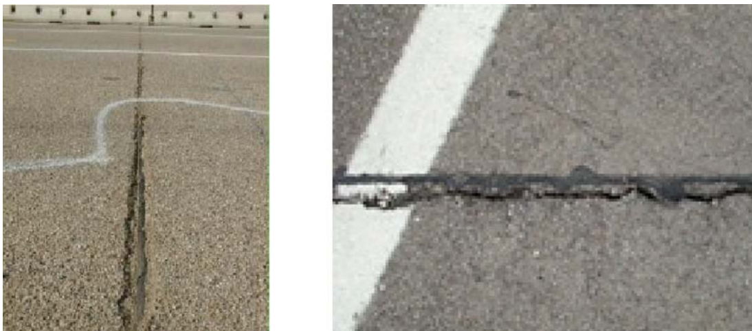
Figure 5.2.1.1-1 Reflective cracking and oozed material at FRP deck-to-deck joints.
