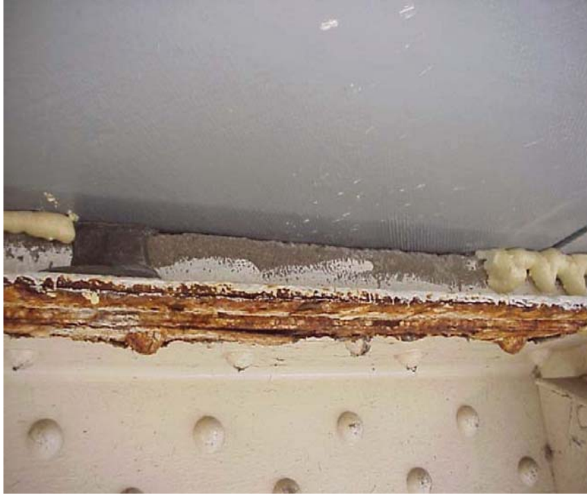
Figure 8-5 Haunch inspection shows deck rise.
