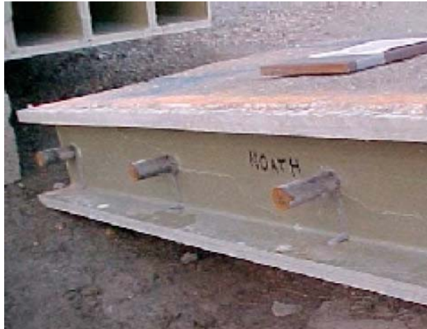
Figure 5.2.1.5-5 Cracks in the web of FRP deck.
