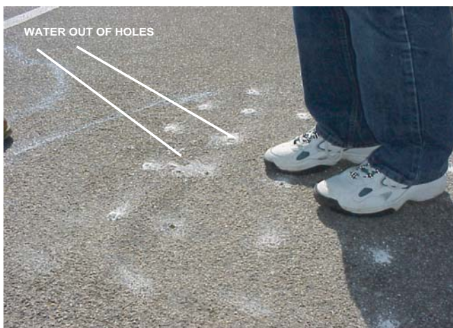
Figure 5.2.2.1-5 Water found within core of deck after drilling.
