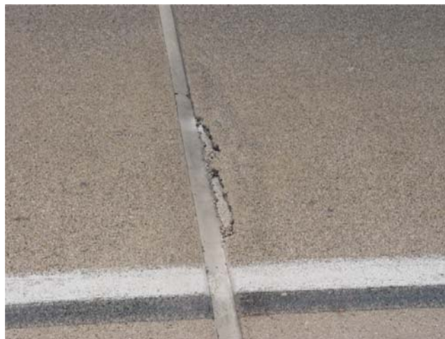
Figure 5.2.1.1-2 Debonding at joint and below wear surface.
