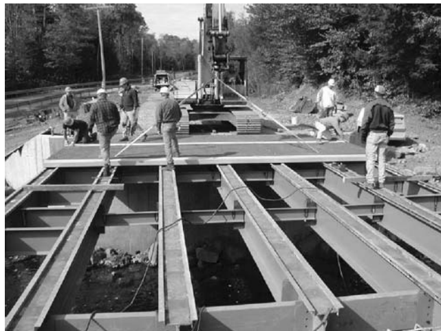
Figure 3.7.3.2.1-2 - Deck being laid down on steel girders; note the channel formed on the top flange for casting haunches.
