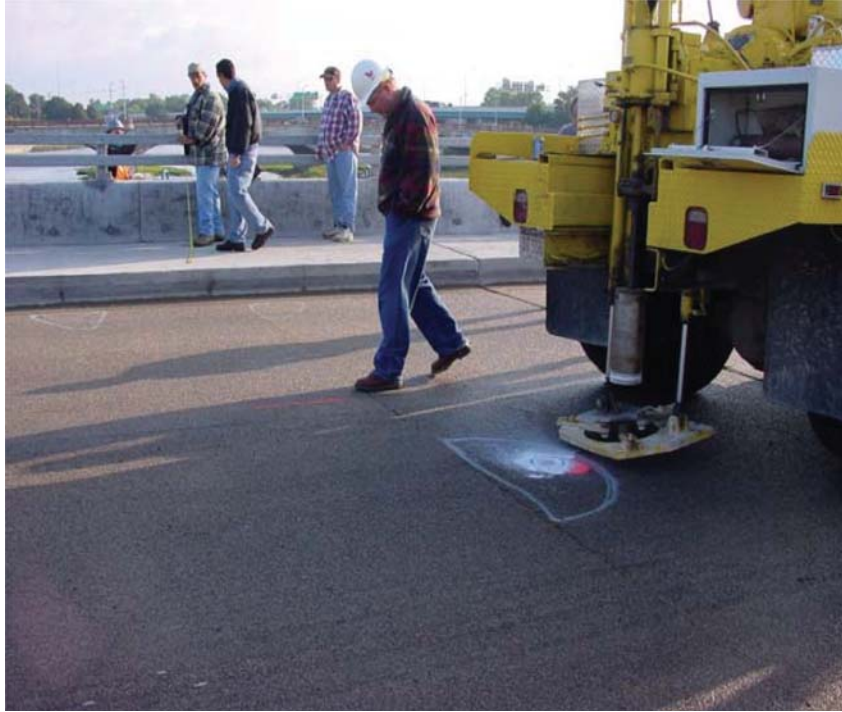
Figure 8-1 Walk-through inspection on Salem Bridge; wear surface cracking and spalling observed.
