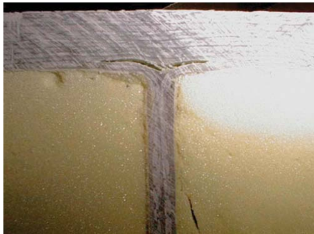
Figure 4.4.2-2 Manufacturing void found in the facesheet of a foam-filled deck.
