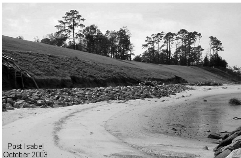
FIGURE 3-17 Overtopping of stone revetment on south side of James River in Isle of Wight County, Virginia. Top of structure is at 2 meters (approx. +8 feet) MLW. Note significant bank scarping due to Hurricane Isabel when the combination of storm surge and wave runup reached 4 meters (approx. +12 feet) MLW. The structure and upper bank face are still intact.
