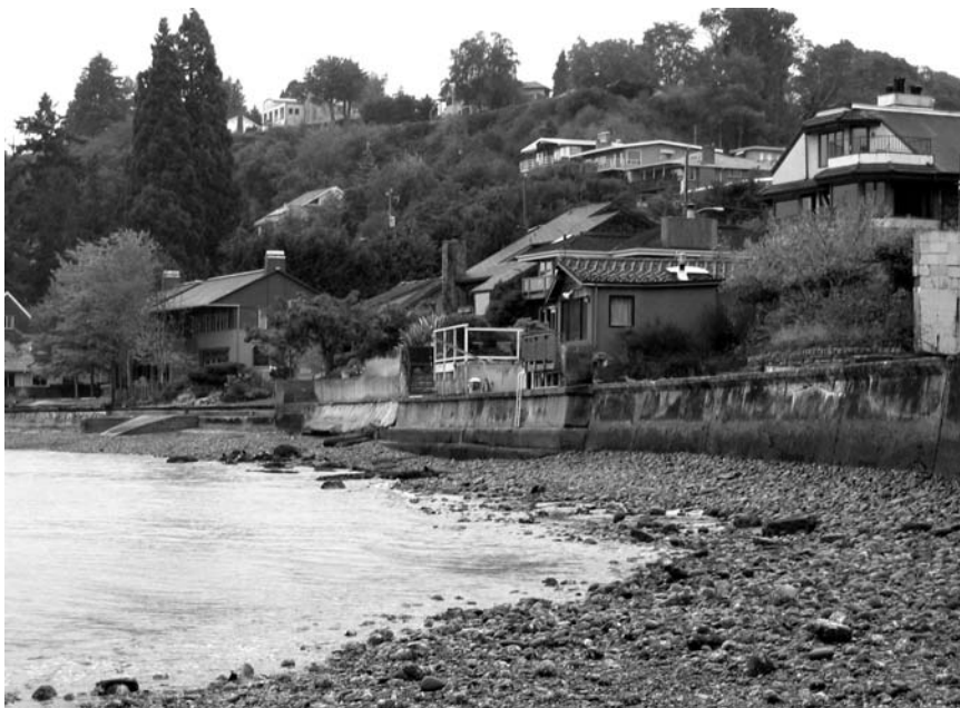
FIGURE 3-5 Concrete seawall in residential area adjacent to Lowman Beach Park in Puget Sound, King County, Washington.
