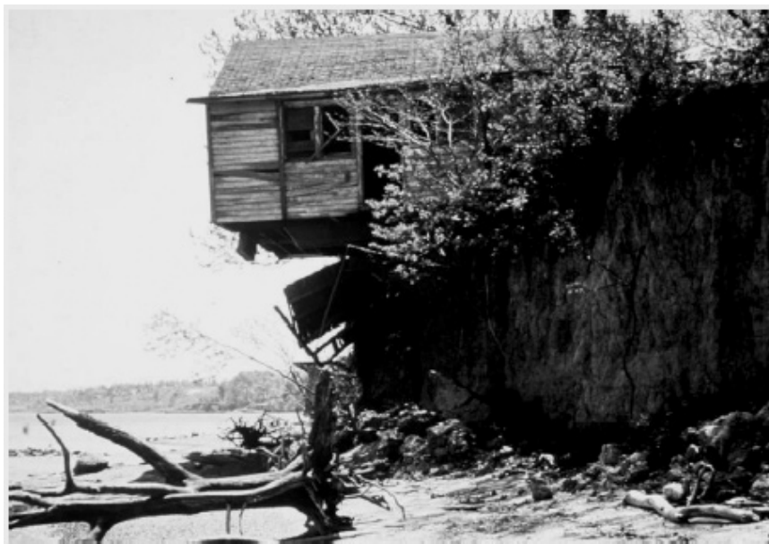
FIGURE 3-16 The result of bluff erosion past the point of being critical. SOURCE: VIMS shoreline photo archive. Courtesy of VIMS.
