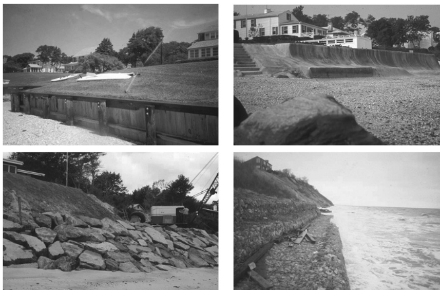
FIGURE 3-3 Shoreline hardening along the coast of Long Island, Long Island Sound. Wood bulkhead (upper left); concrete seawall (upper right); stone revetment (lower left); and gabion seawall (lower right).
