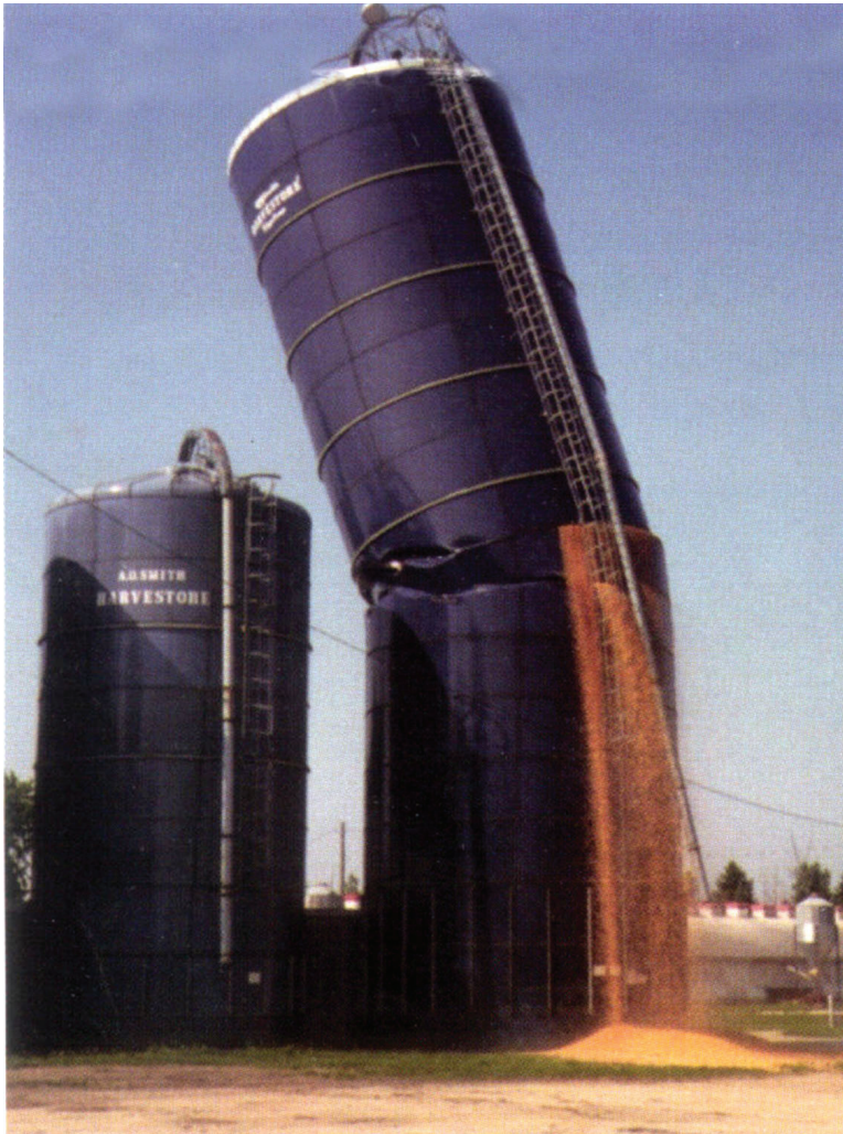
FIGURE 2.7 A collapsing grain silo provides a dramatic example of the unexpected behavior of granular materials. If the grains are flowing in some regions and jammed in others within the silo, there can be large variations of the stress on the silo walls, leading to disaster. SOURCE: J.M.Rotter, University of Edinburgh, and J.W. Carson, Jenike and Johanson, Inc.
