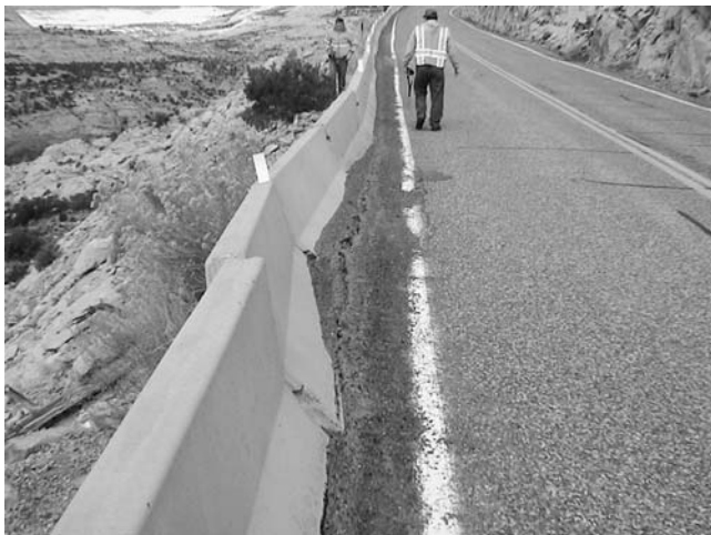
FIGURE 20 Lack of shoulders and washouts along SR-12 project corridor. (Source: UDOT SR-12 project website.)
