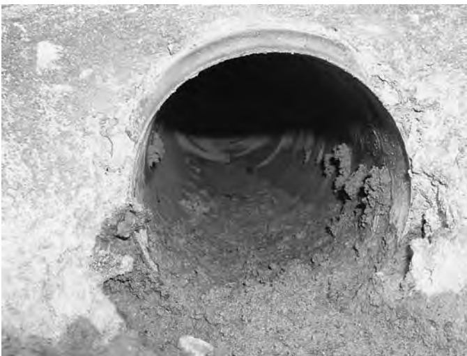
Figure 11. Soil accumulation in drainage outlet at Alabama SPS-1 site.
