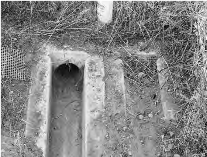
Figure 50. Dual outlets, one cleared for testing, one packed with dirt and stone, Nevada SPS-1.
