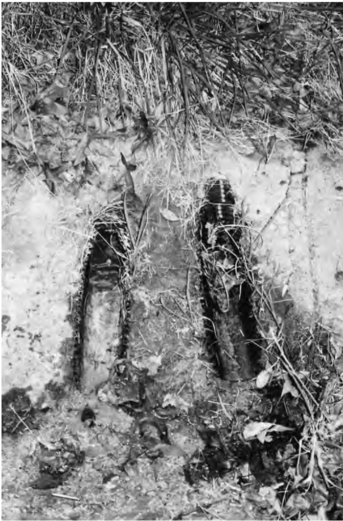
Figure 66. Dual outlets, one flowing, and hardened buildup of past outflow residue, believed to be due to rublizing of old concrete pavement under test sections, Arkansas SPS-2.
