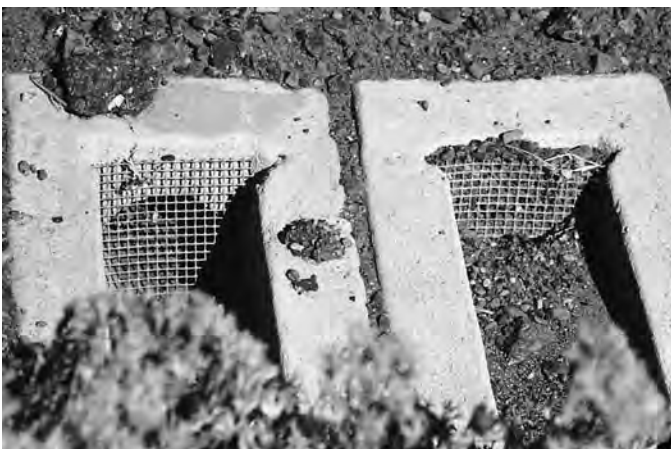
Figure 51. Dual outlets, one cleared, one blocked by dirt and stone, Nevada SPS-2.
