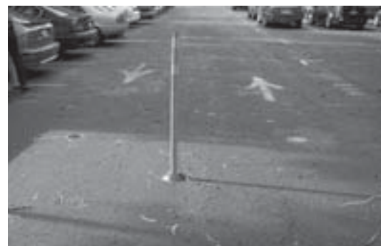
Sensors in the pavement at the parking lot entrance and exit provided a count of space availability.
