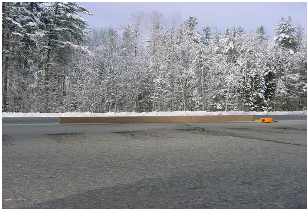
FIGURE 9 Tenting failure of reclaimed Interstate in New Hampshire.
