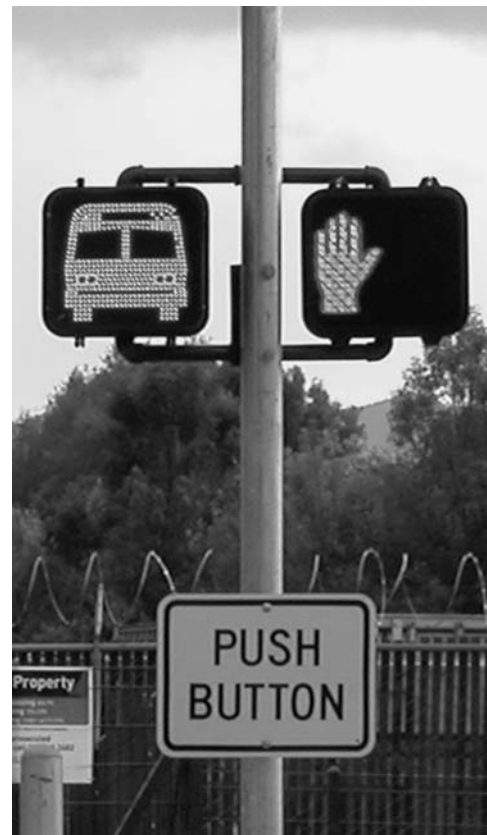
Figure 5-6. Bus-activated warning sign (black with orange symbol) for pedestrian midblock crossings of Orange Line busway, Los Angeles.
