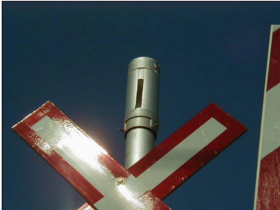
Figure 2. Example of an Electronic Crossing Bell with a Shield (Calgary)
