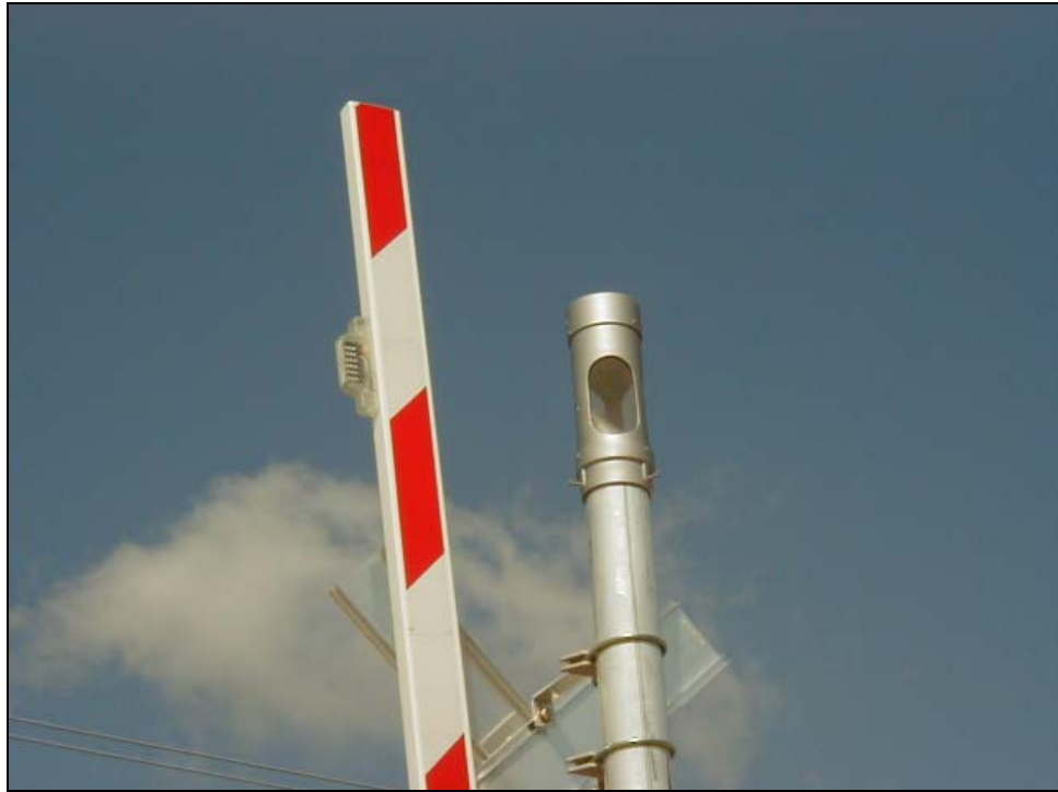
Figure 1. Example of a Typical Electronic Crossing Bell (Calgary)
