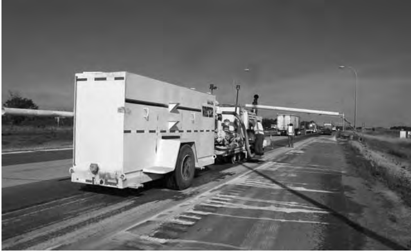
Diamond grinding procedures to restore the ride and texture of concrete pavements are tested and evaluated at MnROAD.
