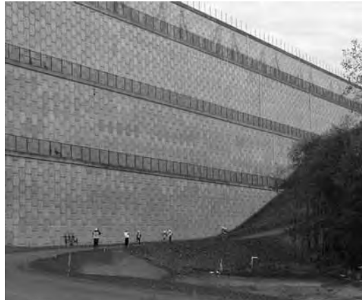
The 140-ft high MSE wall at Seattle-Tacoma International Airport allowed for a critically needed third runway.
