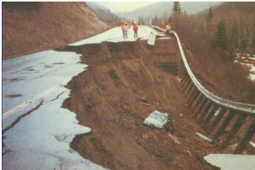
FIGURE 1 Recurring landslide on Colorado State Highway 133 at McClure Pass, west of Aspen, in spring 1993—a good reason for research.
