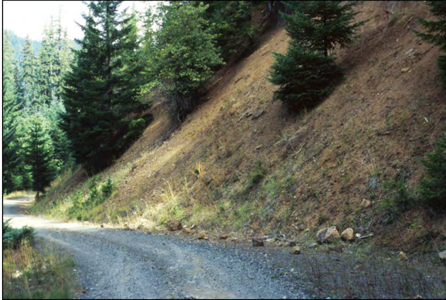
An unpaved forest road in steep terrain with a large cutslope. Photo courtesy of B. Wemple.
