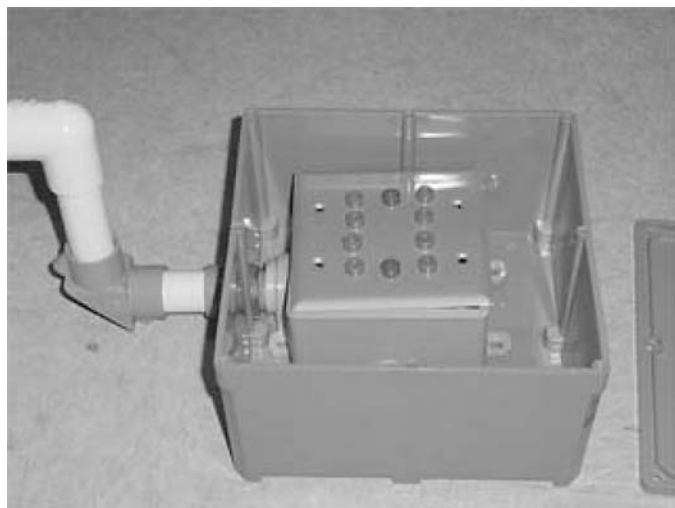
Figure 4.27. PVC connection box and connectors.
