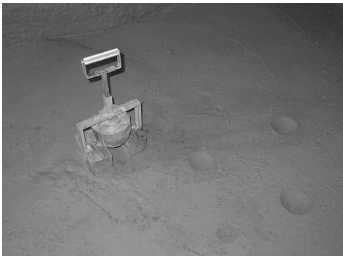
Figure 4.18. Use of Kelly ball to determine the proper timing of hot-mix asphalt paving.
