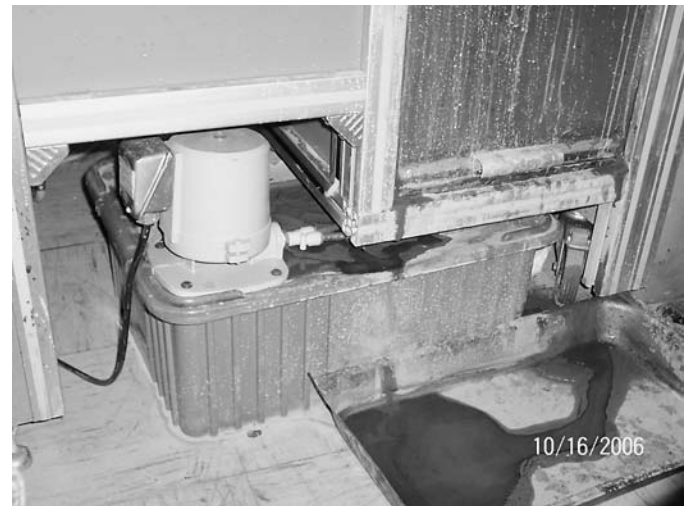
Figure 33. Water circulation system.
